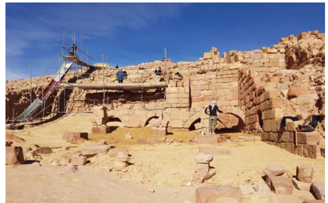
Nearing completion of the backfilling in the SW Quadrant in mid-December (photo Jack Green)
