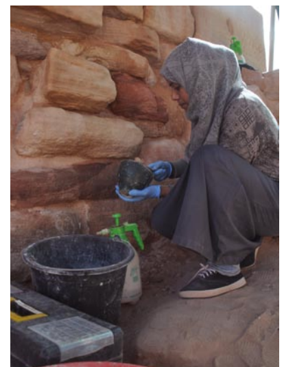
Conservation trainee Ghadeer Jdeilat applying a new layer of mortar between the stones of the cella's south wall (photo by Halemah Nawafleh)
