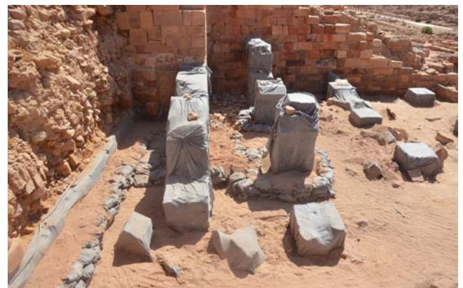
The architecture of the temple's deep southwest quadrant wrapped in gray geotextile and buttressed with soil and protective sandbags to prevent the accumulation of damaging moisture once the area is backfilled (photo by Eman Abdessalam)
