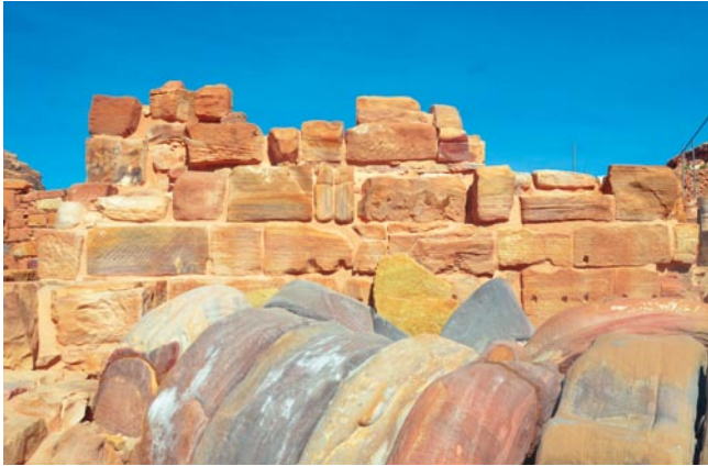
Exterior face of the cella's southwest wall after completion of conservation treatment and application of final mortar layers (photo by Eman Abdessalam)
